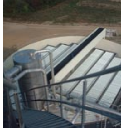
Industrial effluent treatment at Nakskov sugar mill, Denmark.
