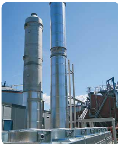
Linköping, Sweden, 3450 Nm 3 /h, 2030 scfm.
