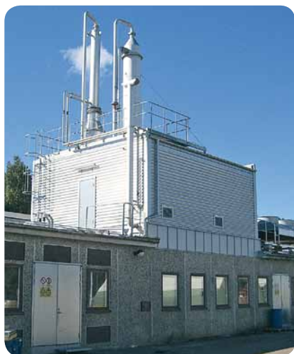
Gothenburg, Sweden, 1600 Nm 3 /h, 930 scfm.
